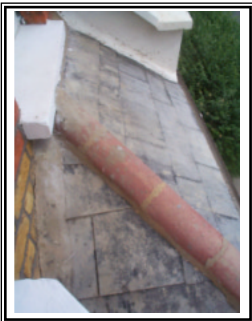
Photo 7 – Staining to porch roof
