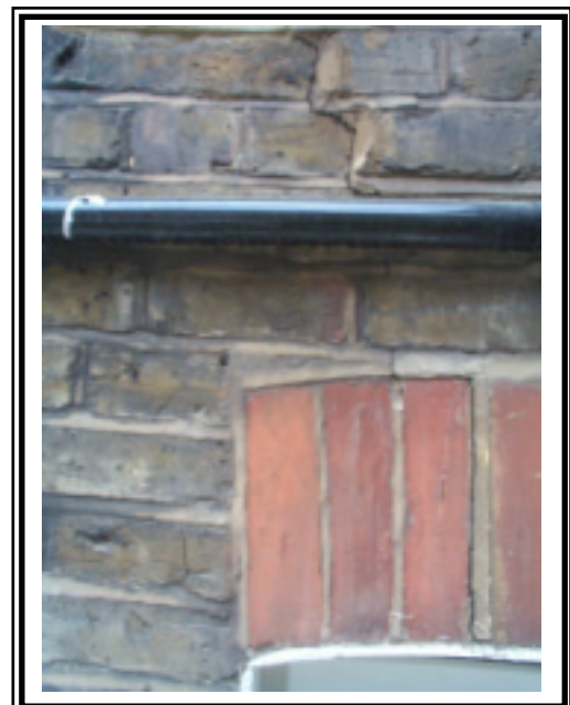
Photo 4 – Cracking over bathroom window
